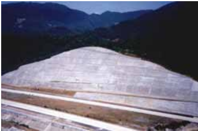
Fig. 1 A section of ↑ highway and its huge “scar” being constructed in northern hilly region of Guangdong
