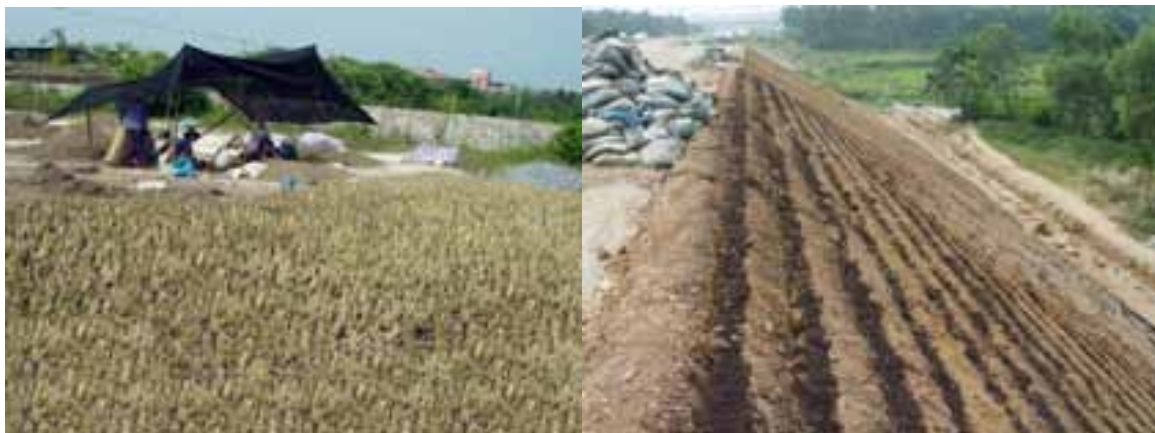
Fig. 7 The first vetiver project conducted on the highway with the new variety, Karnataka Left: preparation of ploybag vetiver seedlings Right: level ditches and basal manure applied prior to planting vetiver
