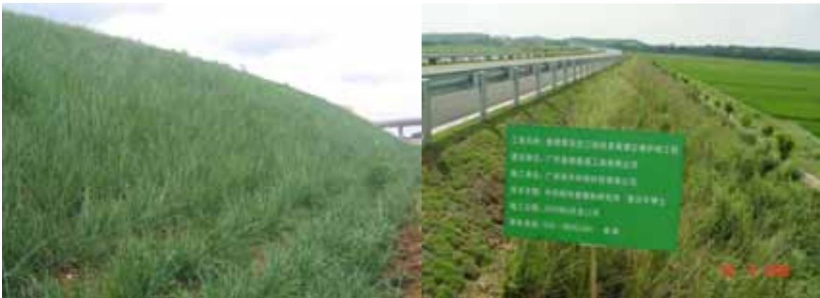
Fig. 9 Left: a upper cut covered and stabilized by hedgerows of Karnataka vetiver Right: a wonderful vista composed of the highway itself and vetiver hedge-belt rounding it
