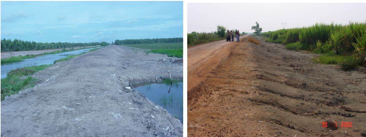
Photo 1: Severe erosion on canal and rural road on Acid Sulfate soil
